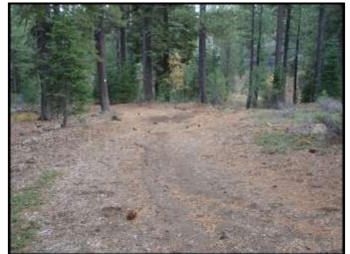
Photo 11b – Typical Road Surface and Rolling Dip w/ Dissipater Improvement
