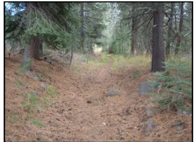
Photo 20d – Rolling Dips w/ Dissipaters Improvement Typical of Existing Roadbed Segment of Project
