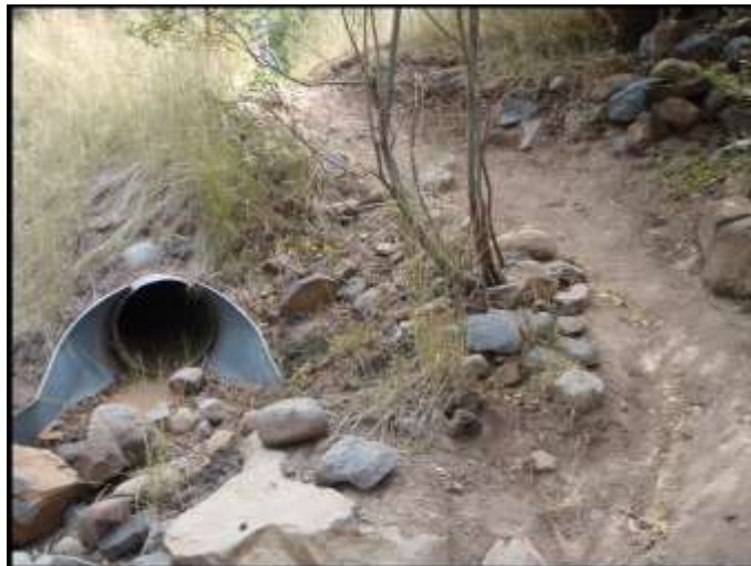
Photo 22e – Area of Rock Steps Installation of Segment 22C on Downhill/North Side of Brookstone Drive
