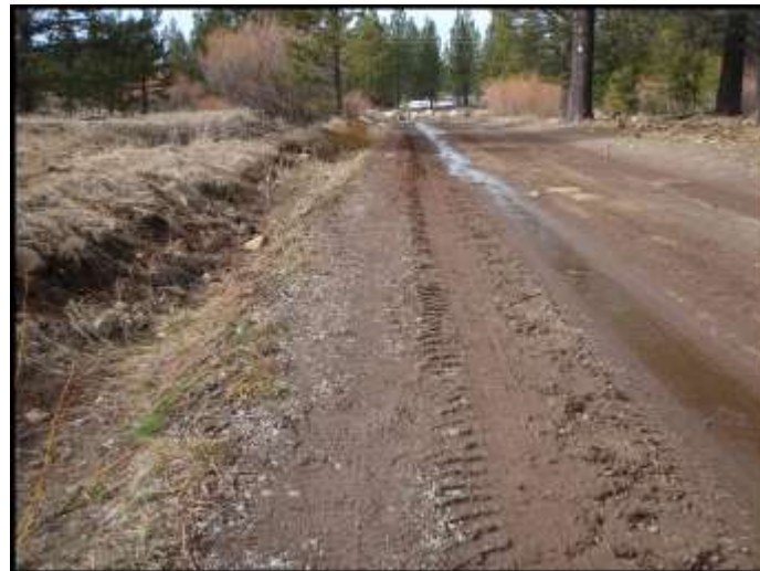
Photo 1e – Road Re-Surfacing & Stabilization Near Project Start at end of Alder Creek Road
